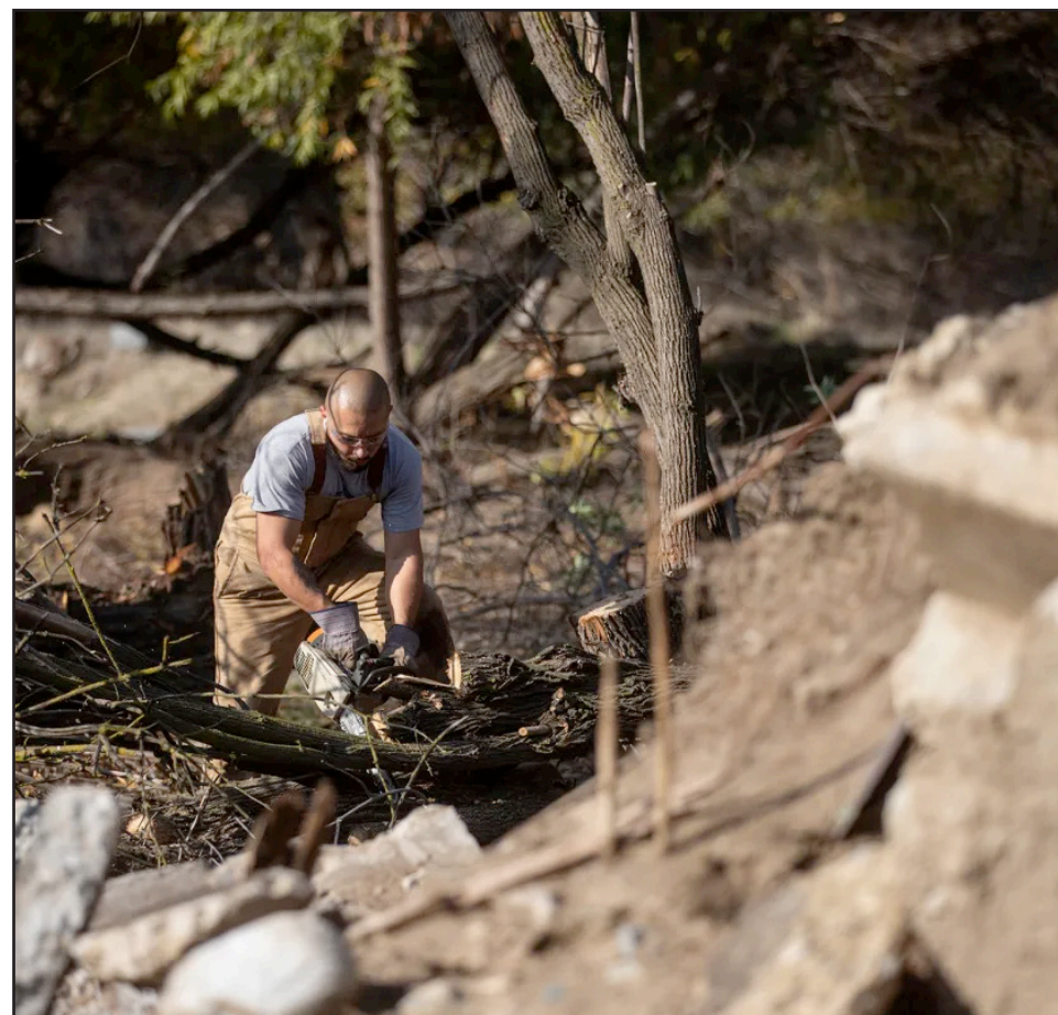
Temporary worker Demetrius Ensign uses a chainsaw to cut tree branches and trunks in Bartlett Park in Porterville on Dec. 4, 2024. Workers from the National Dislocated Worker Grant, a federally funded jobs program, are helping to clean the park of flood damage. Photo by Larry Valenzuela, CalMatters/CatchLight Local
